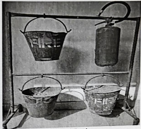
Fire Sand Buckets
